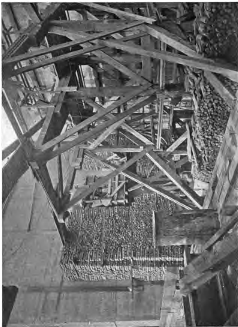
PLATE 233. —Contract 67. Shaft 21. Sinking of Wall Caissons for Enclosing Area above Shaft. Showing pig iron piled on top of caisson to overcome friction against gravel.
